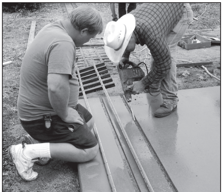
Grooves to hold the miniature-train track are cut in the station-platform concrete by Harry Vanderhoofven, with assistance from Tom Brown (left), father of Junior Engineers Jordan and Matt Brown.
