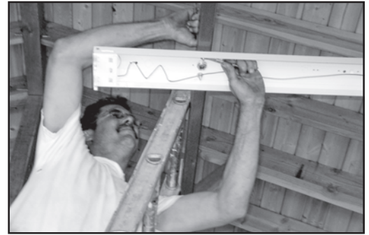
The Visitor Center has lights! Ron Koens installs one of the fixtures, July 30, 2005.
