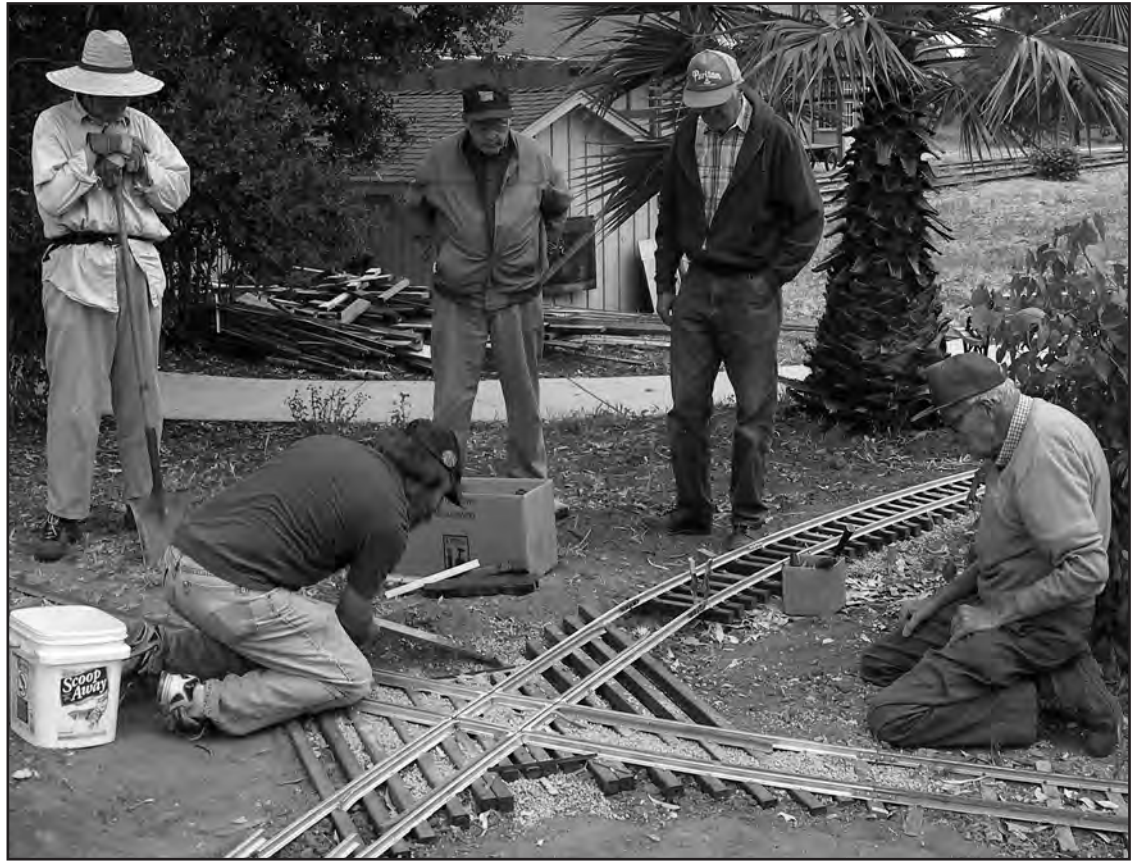
Bruce Morden, foreground left, works on one of the new crossover tracks, while Gene Allen, right, supervises. Standing, left to right: Ed Leska, Bern Verbit, and John Green.
