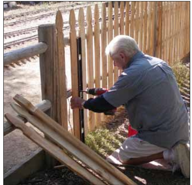
Volunteer Tony Ramirez installs pickets near the Goleta Short Line passenger entry gate.
