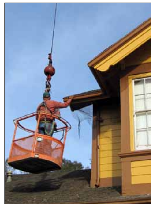
Finishing touches on bird-netting installation by Gary Coombs and Doug Winter required boom-truck services, donated by Specialty Crane & Rigging (photos by Ed Leska).
